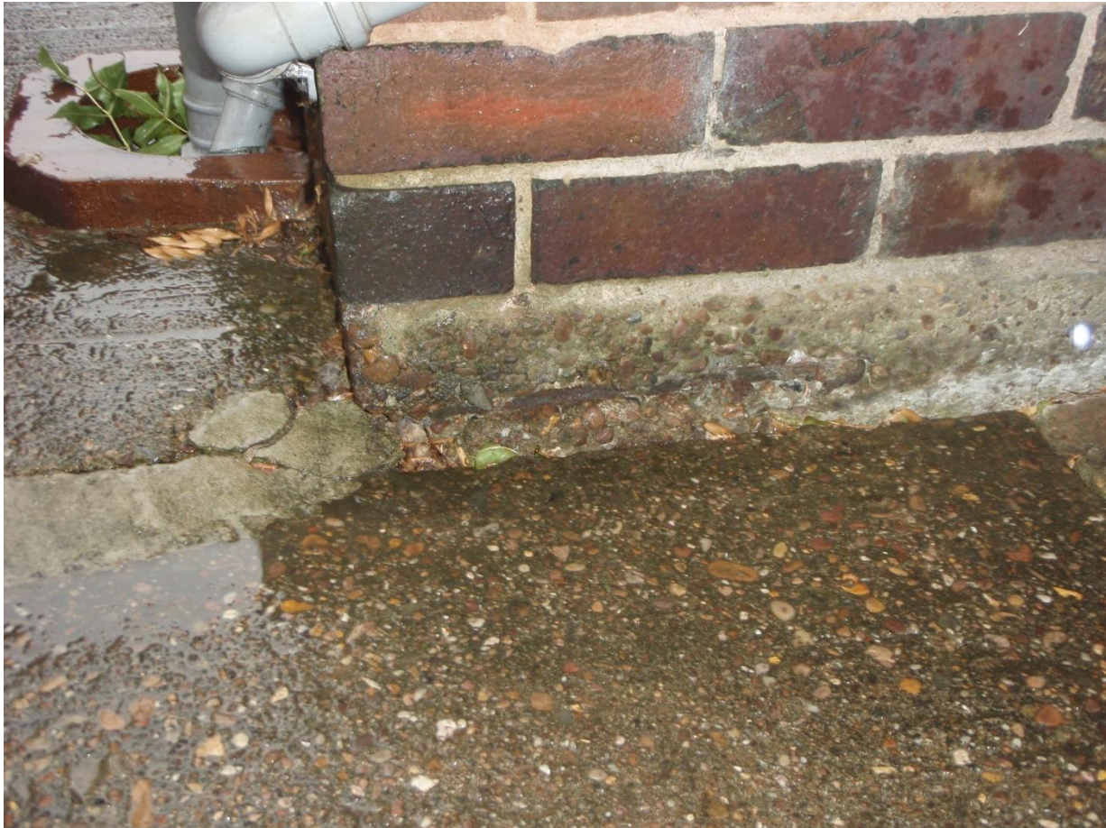
EXPOSED CORRODING REINFORCEMENT IN RAFT FOUNDATION
