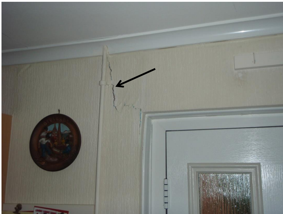
CRACKS OVER REAR KITCHEN DOOR
