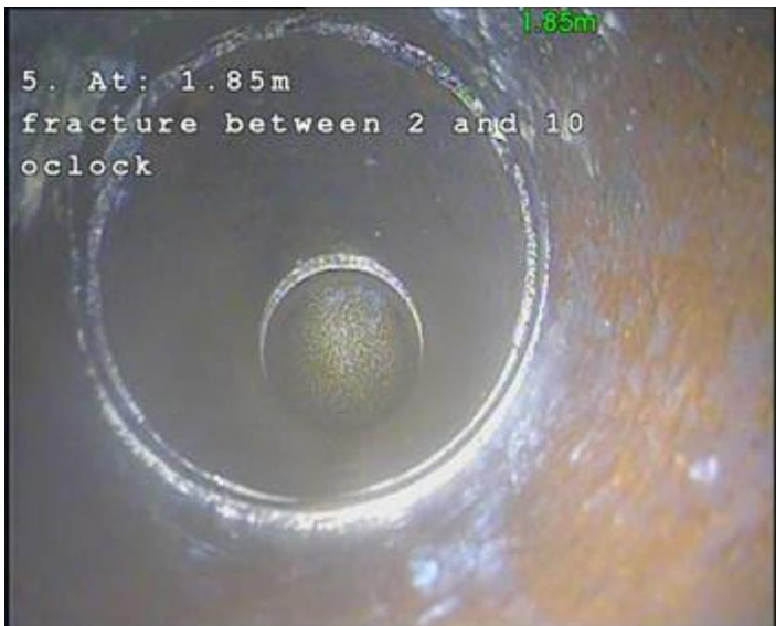
5. 1.85m Fracture between 2 and 10 o'clock
