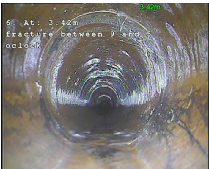
6. 3.42m Fracture between 9 and 5 o'clock
