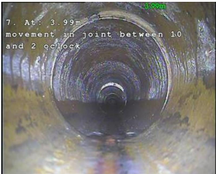
o. 3.99m Displaced joint between 10 and 2 o'clock
