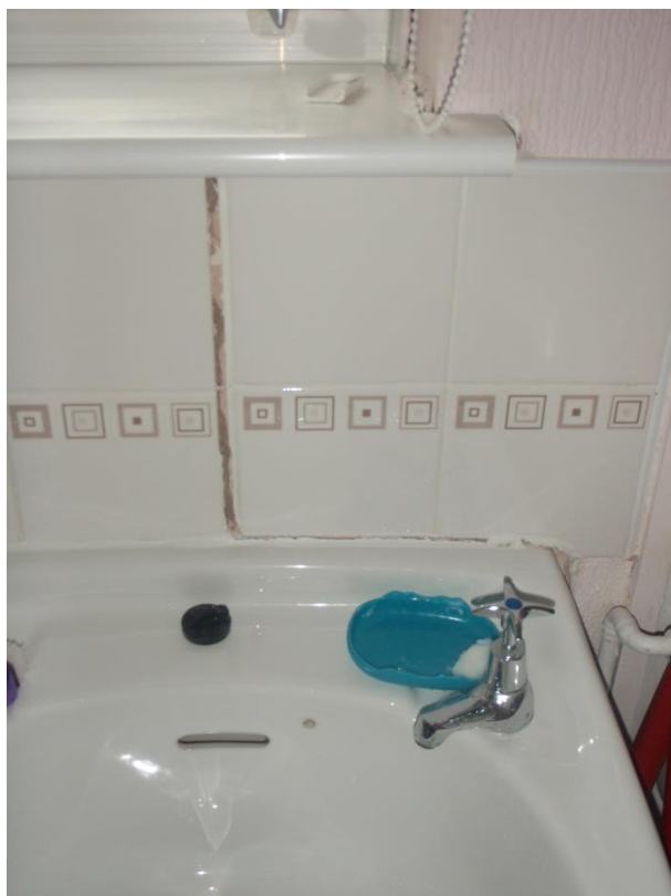
VERTICAL SECTION OF CRACK UNDER BATHROOM WINDOW
