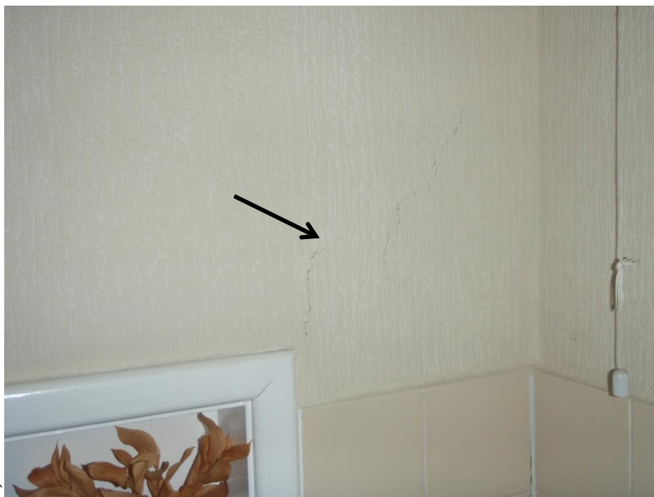
CRACKING OVER KITCHEN SERVING HATCH
