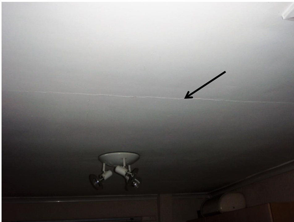
CRACKS IN KITCHEN CEILING
