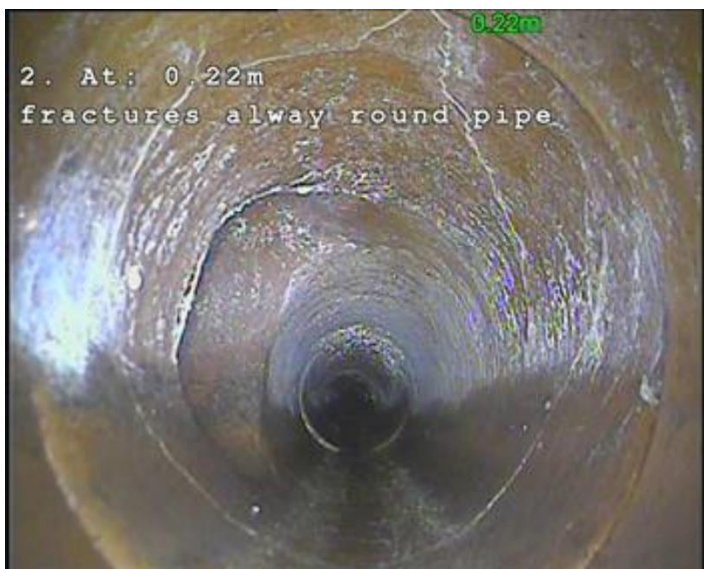
2. 0.22m Circumferential fractures
