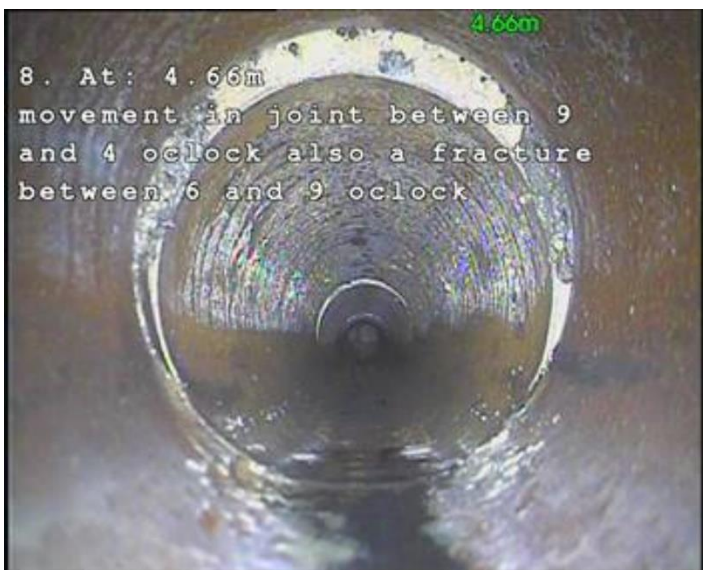
o. 4.66m Displaced joint between 9 and 4 o'clock also a fracture between 6 and 9 o'clock
