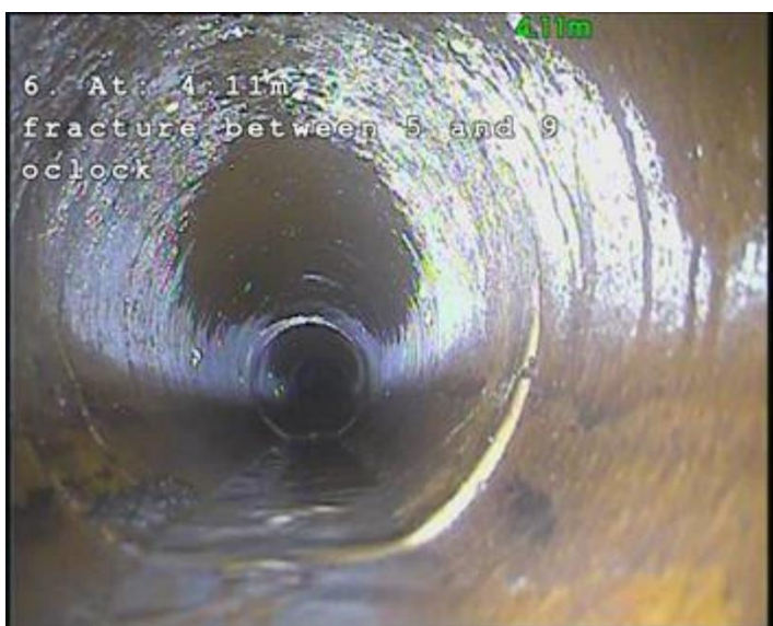
6. 4.11m Fracture between 5 and 9 o'clock
