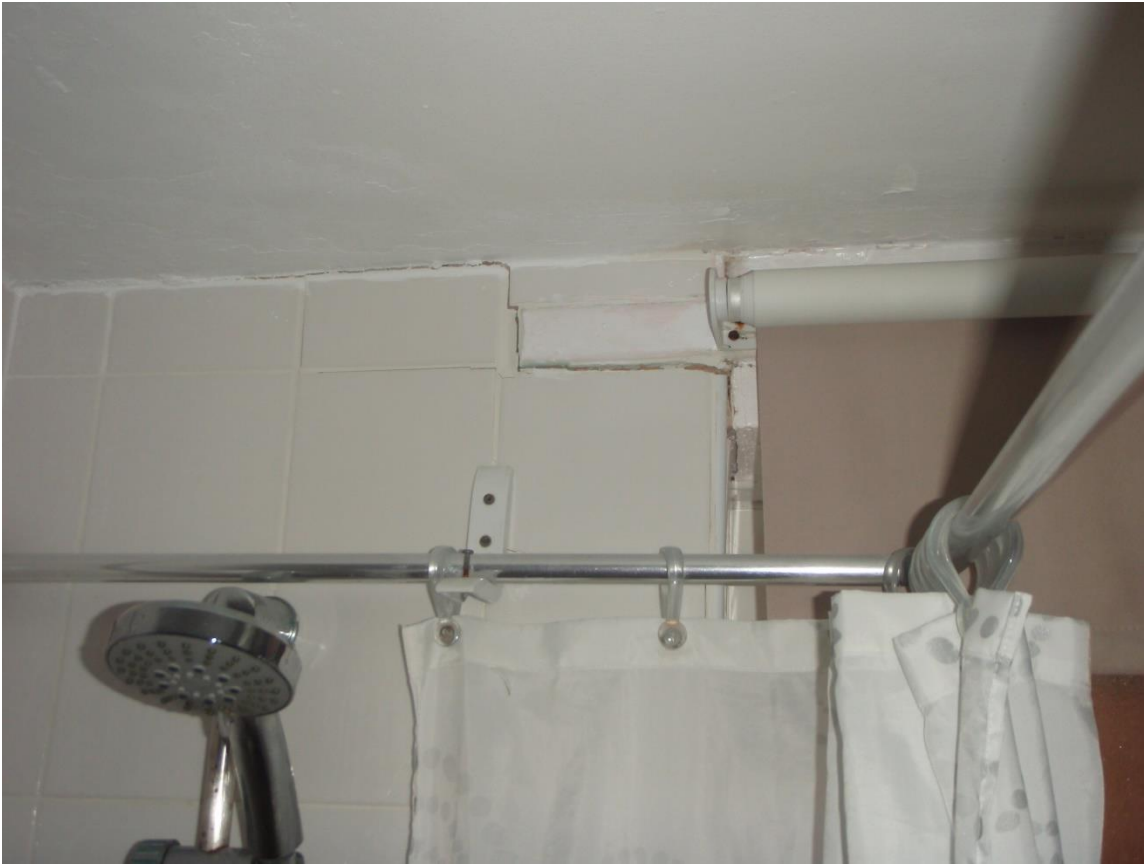
CRACK IN EXTERNAL BATHROOM WALL AT TOP OF WINDOW
