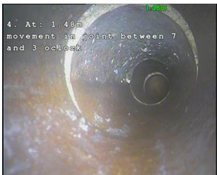
4. 1.48m Displaced joint between 7 and 3 o'clock
