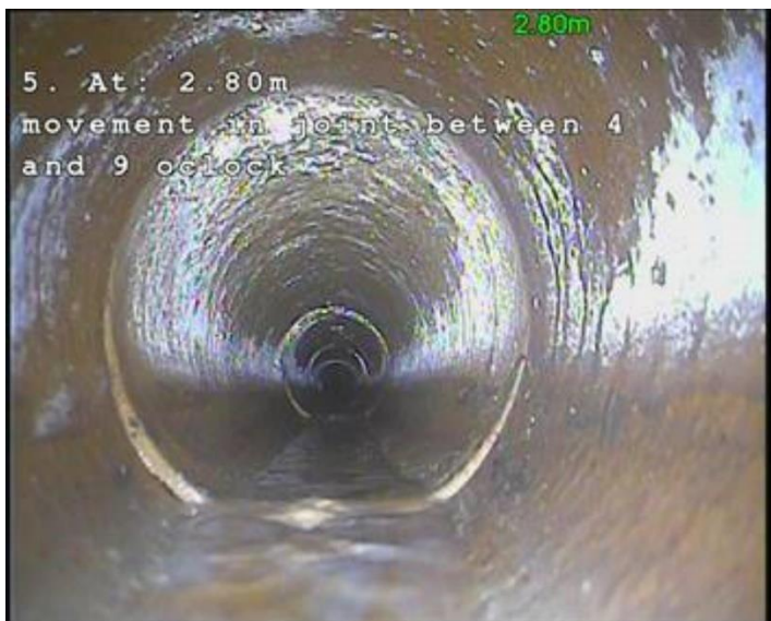
5. 2.80m Displaced joint between 4 and 9 o'clock
