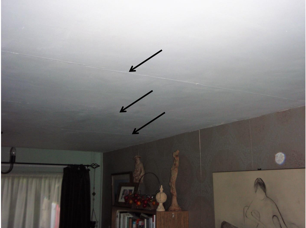
CRACKS IN LOUNGE CEILING
