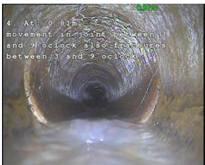
4. 0.81m Displaced joint between 3 and 9 o'clock also fractures between 3 and 9 o'clock
