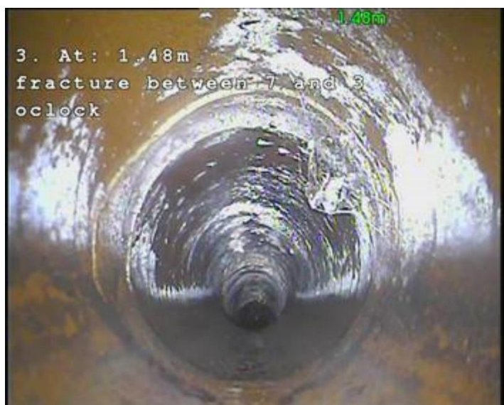
3. 1.48m Fracture between 7 and 3 o'clock
