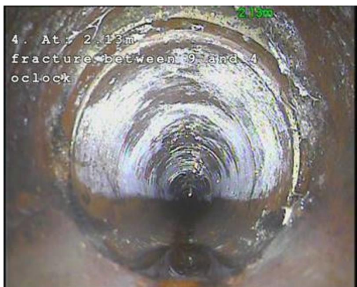
4. 2.13m Fracture between 9 and 4 o'clock
