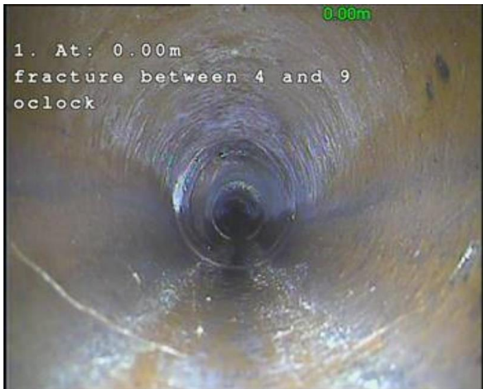
0. 0.00m Fracture between 4 and 9 o'clock
