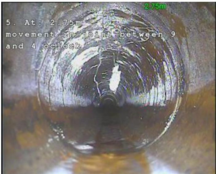
5. 2.75m Displaced joint between 9 and 4 o'clock
