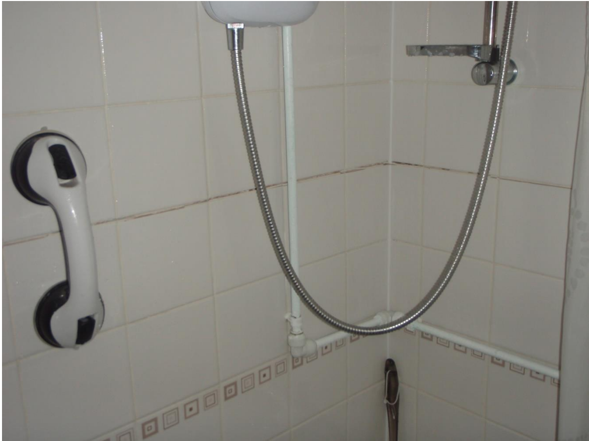
HORIZONTAL CRACK IN BATHROOM WALL
