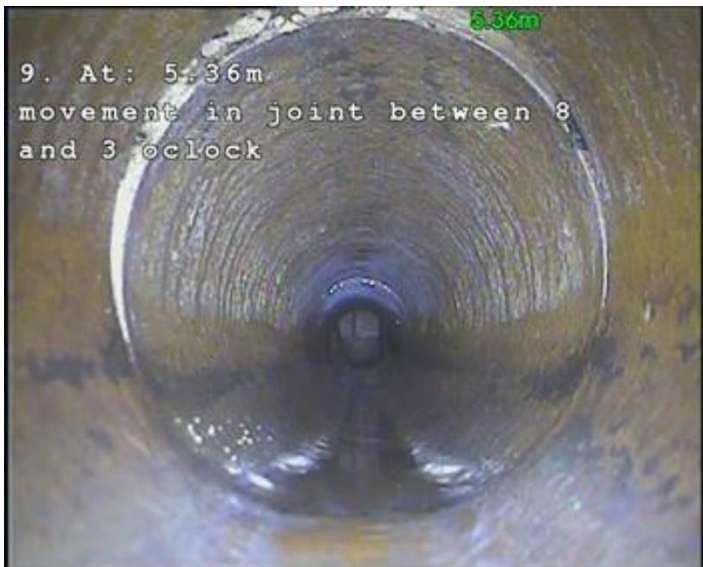
9. 5.36m Displaced joint between 8 and 3 o'clock
