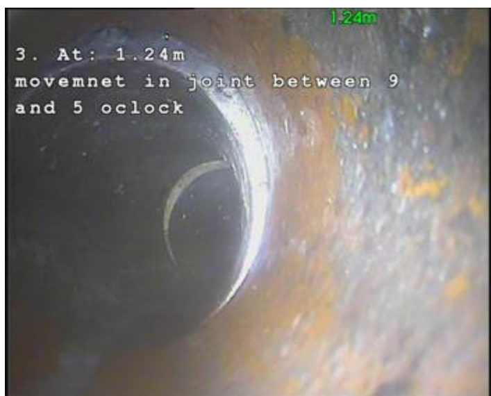
3. 1.24m Displaced joint between 9 and 5 o'clock
