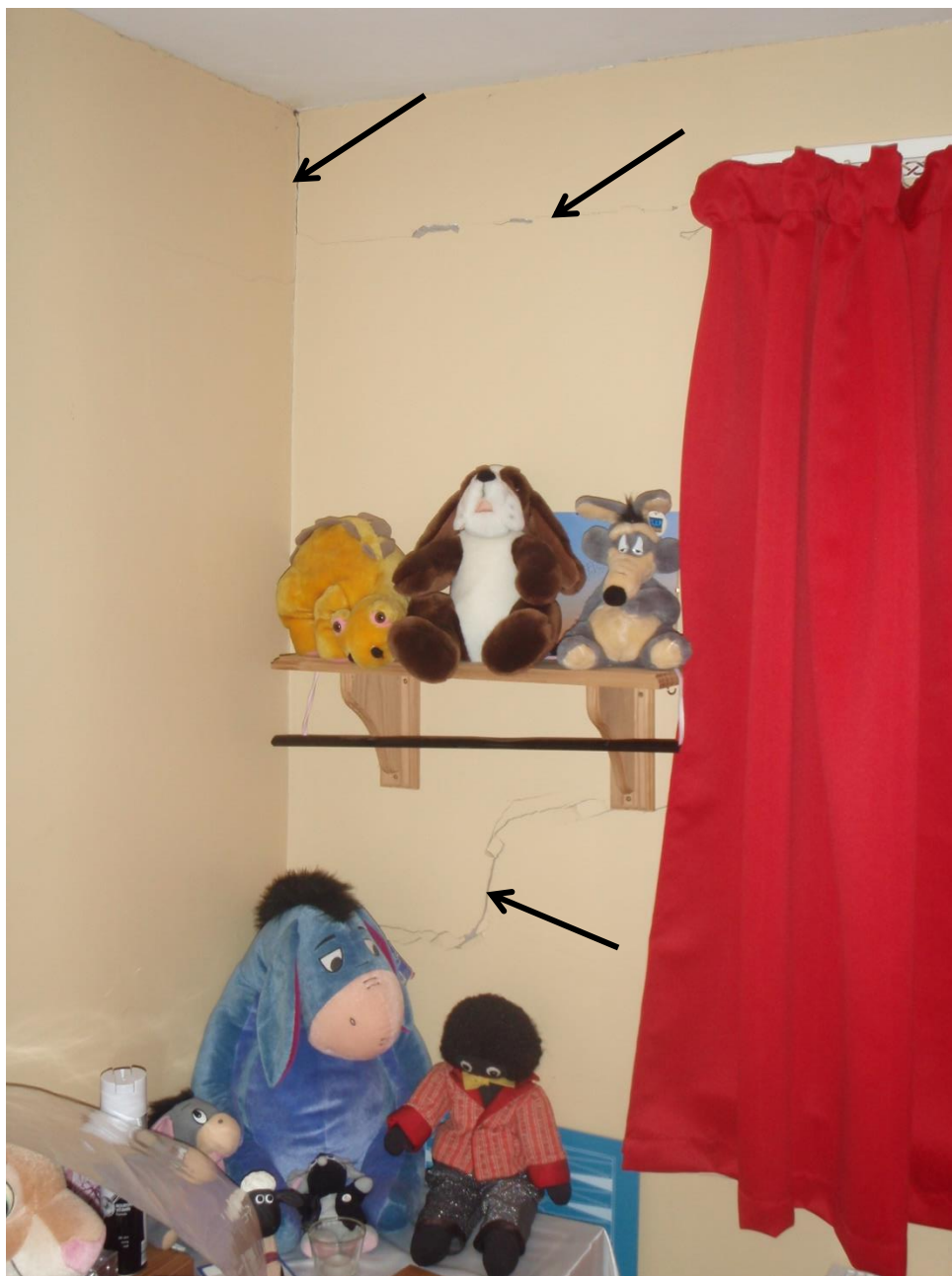
HORIZONTAL AND DIAGONAL CRACKS TO REAR WALL SMALL BEDROOM
