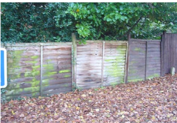
Visually detracting timber fencing
