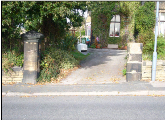
Loss of copings on a gate pier
