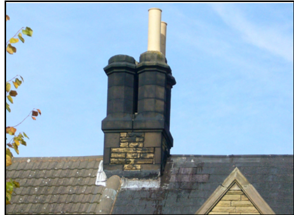
Loss of chimney pots
