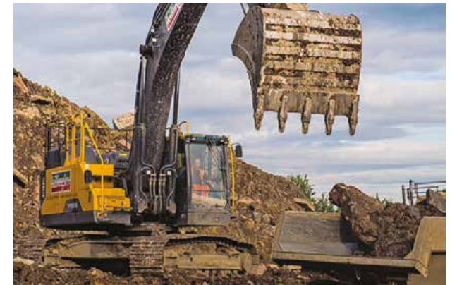
Preparatory work has already started on the Basin Square Phase of the Waterside scheme
