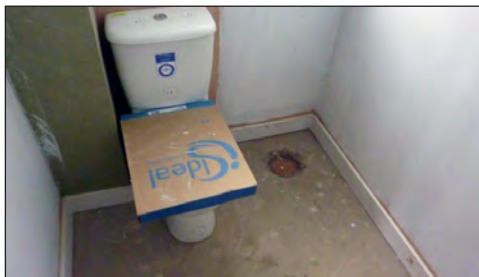
Lifetimes Homes in practice - a cloakroom with pre-installed drainage to allow later conversion to a wet room
