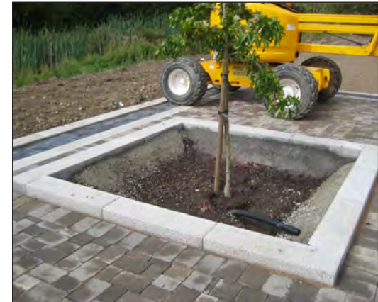
A properly designed and constructed tree pit means that the tree will have a greater chance of becoming established and a long term addition to the street scene
