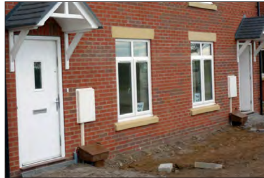
Meter boxes prominently positioned on front elevations detract from the appearance of these houses
