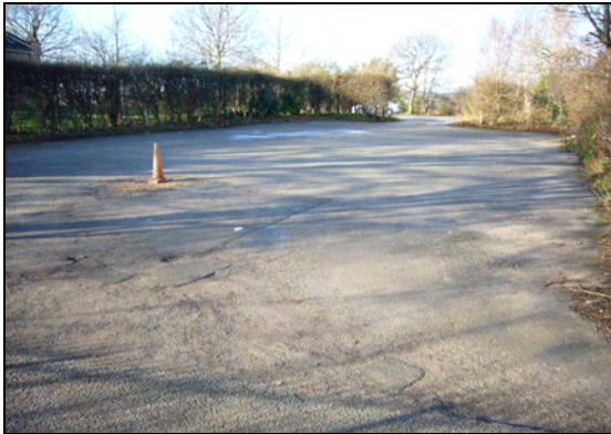
Poor maintenance Nag's Head car park
